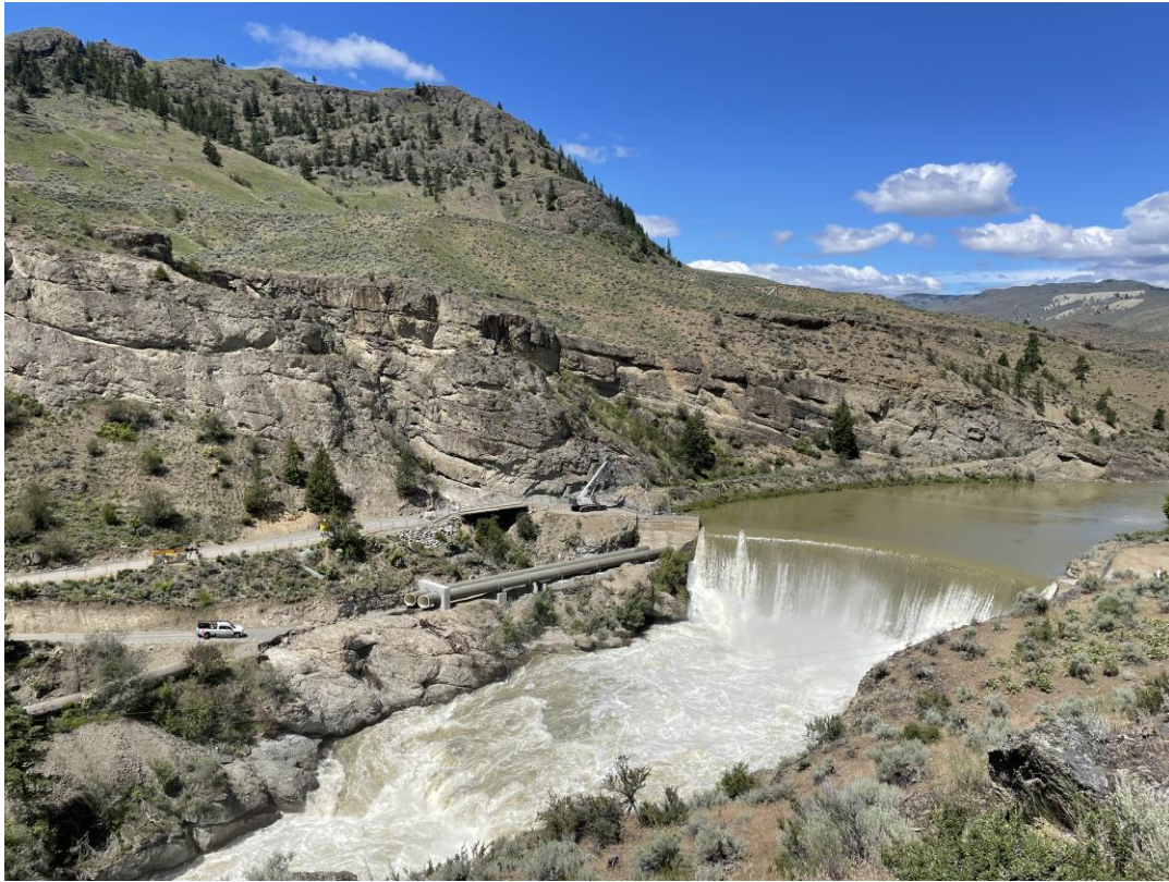
Figure 19. Enloe Dam on the Similkameen River lies a short distance upstream of Coyote Falls, near the truck parked by the dewatering pipes that have been constructed along the right bank.
