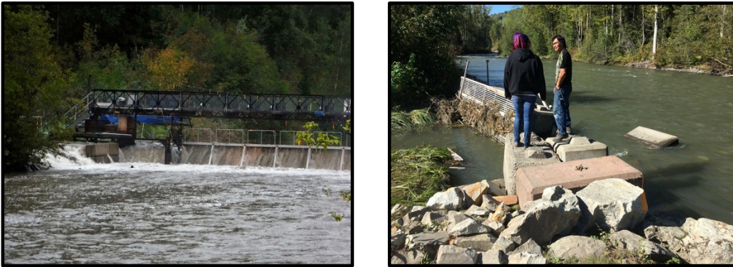
Figure 21: High water on September 11 th , 2017 - right bank (left) and damage to outlet of side channel (right).
