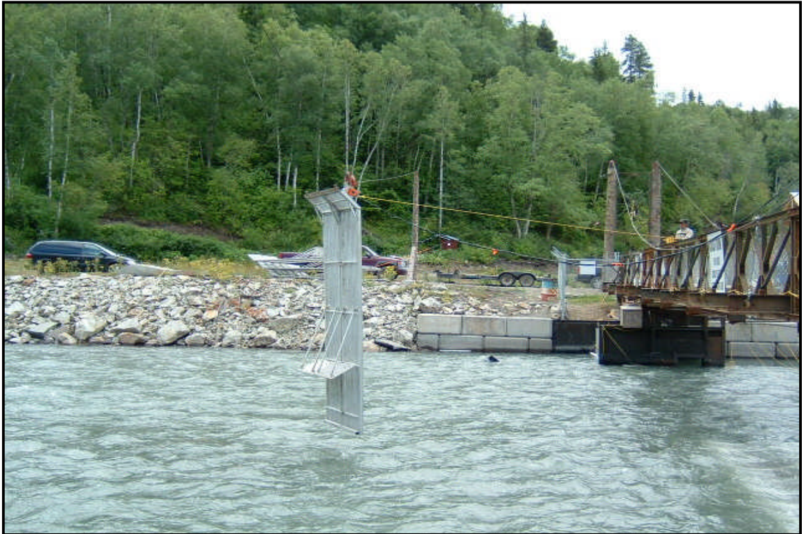
Photograph 3. Overhead winch used to lower and raise aluminium panels in and out of the river.
