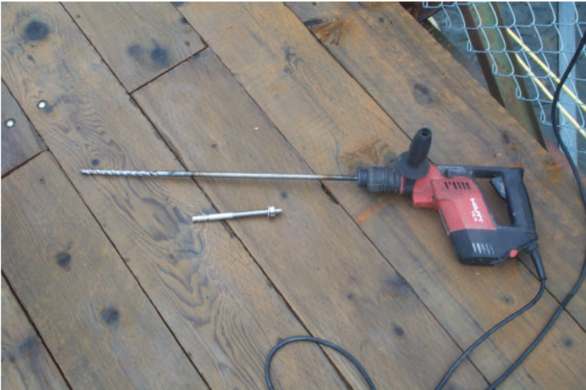
Photograph #1: Hilti Drill, specialized drill bit and Hilti stud used to secure fence hooking bracket to cement crump.
