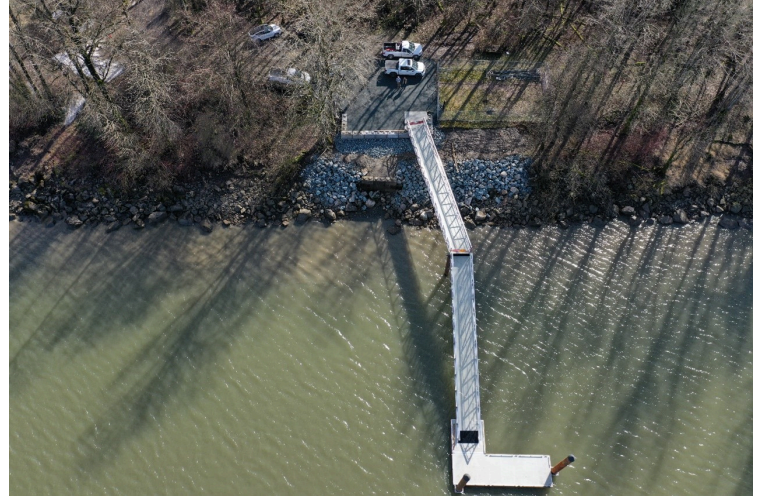
Aerial view of the floating dock, bank remediation and crane pad during commissioning February 2025
