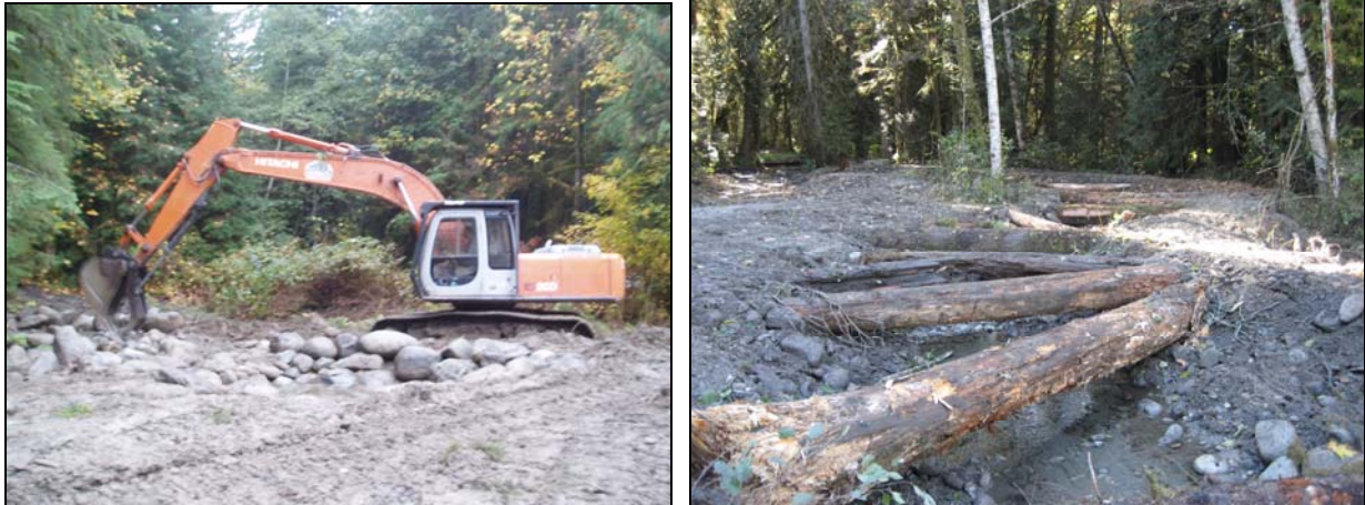
Figure 3 Placing rock in spawning channels (a) and large wood added to channels (b)
