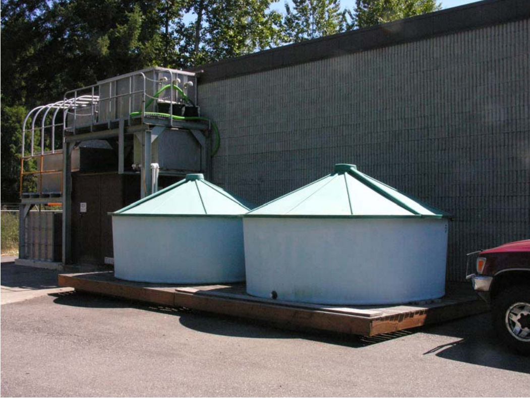
Figure 29. Tanks 5 and 6 (10-ft diameter at Puntledge Lower Site) ) showing extra aeration head tank.
