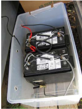
Batteries used to provide power to computer, cameras and peripheral gear.
