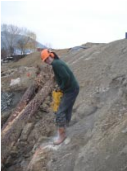
Cables holding logs were anchored to the bank
