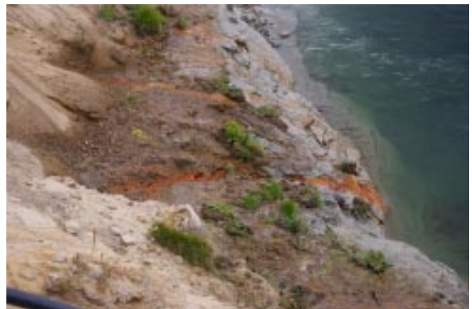
Ground water exiting bank
