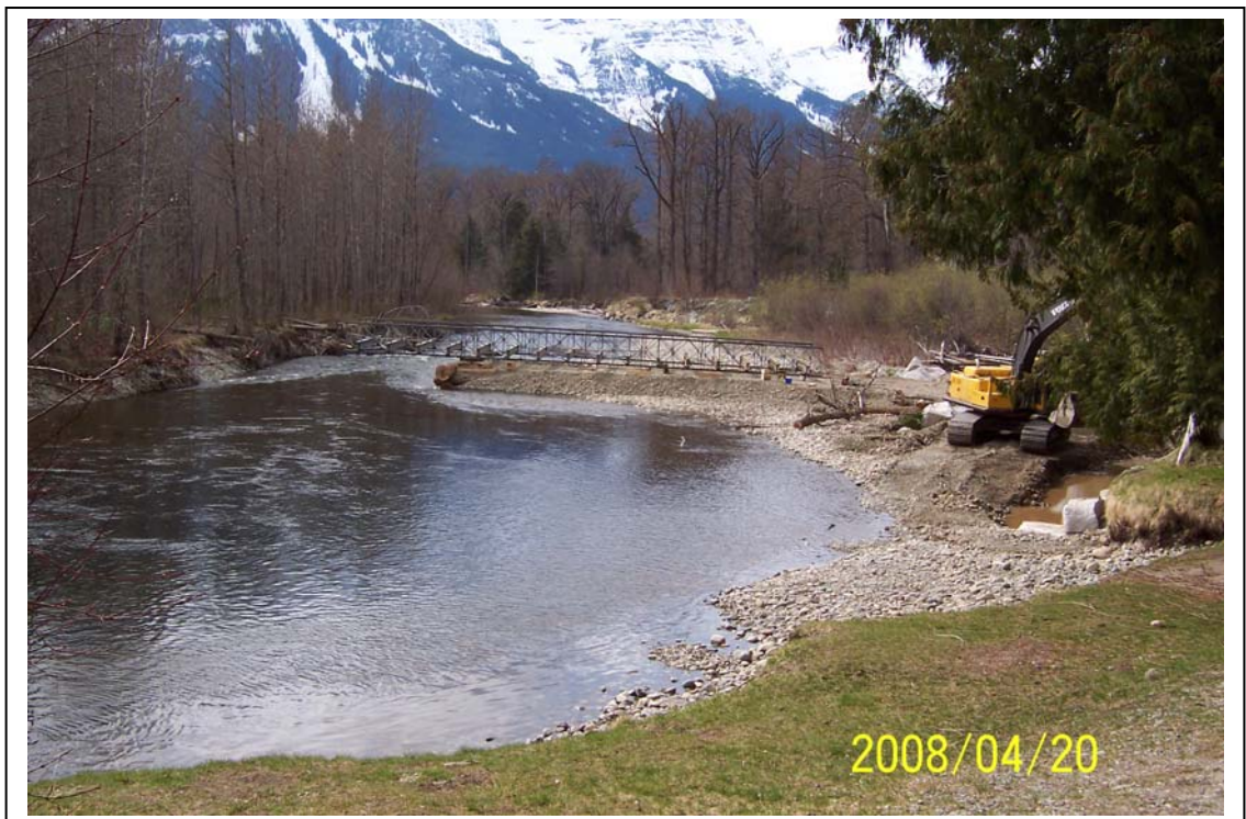
Figure 3. Bridge construction across the Atnarko River, excavator is beginning intake channel reconstruction and rock armor placement.
