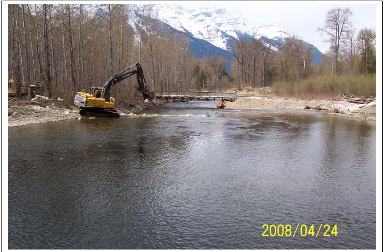
Figure 4. Excavator placing rock deflection groyne against river bank opposite the intake channel.
