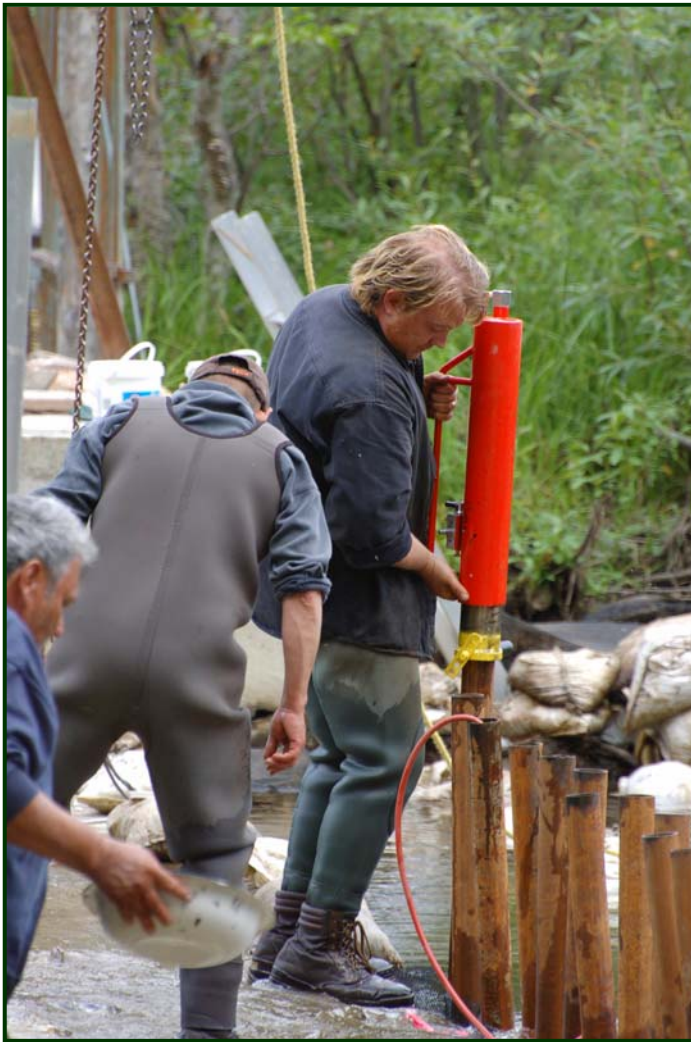
Figure 6. Placement of steel drill pipe sections along the downstream edge of the weir, August 2008.
