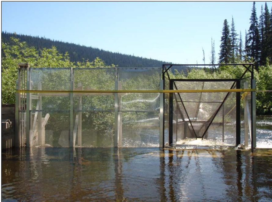
Figure 5. View downstream of newly constructed fyke trap (#2) opening and adjacent perforated panels from the bank left pier.
