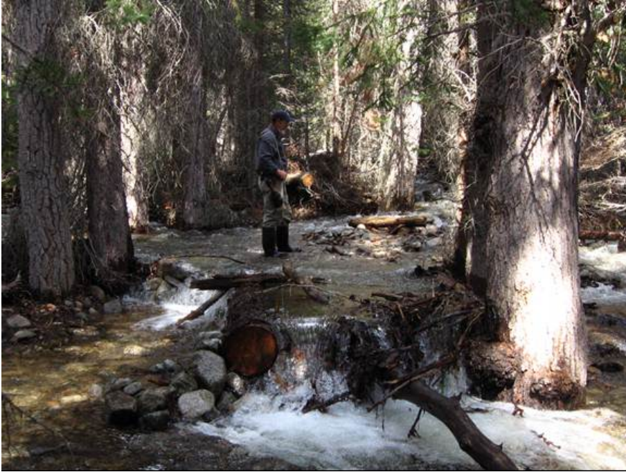
Figure 3. Dam and water impoundment structure after flood event.
