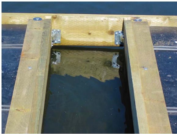
Figure 3. Simpson Strong-Tie galvanized reinforcing angles were used to connect the structural members. Note attachment of float units on right and left.
