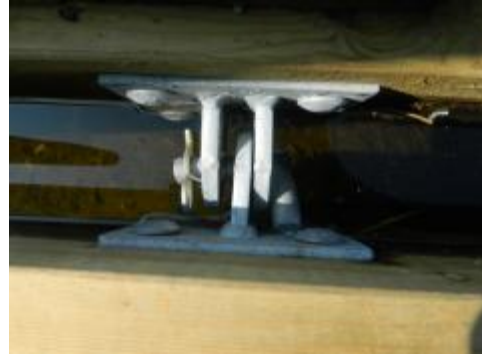
Figure 2. One of two heavy-duty hinges joining the two sections of the dock.
